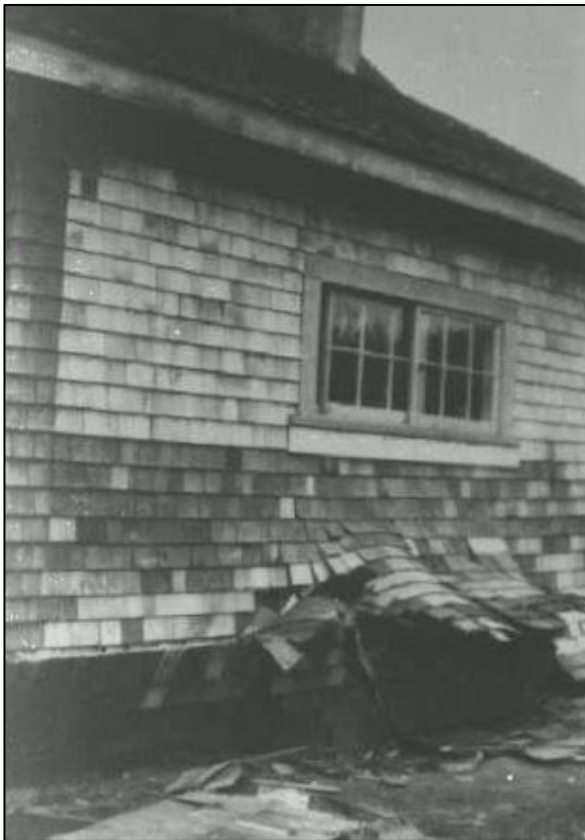
Figure 1 Foundation failure in Comox, 1946 earthquake
