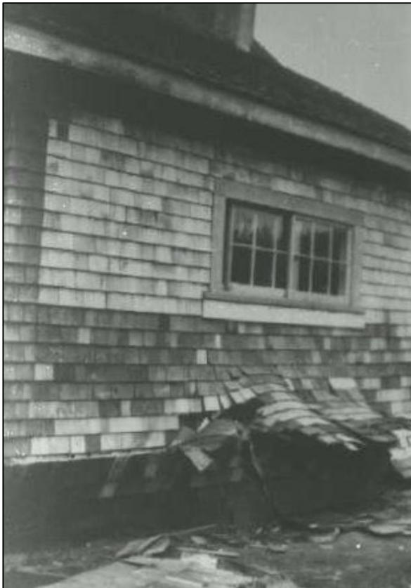
Figure 1 Foundation failure in Comox, 1946 earthquake
